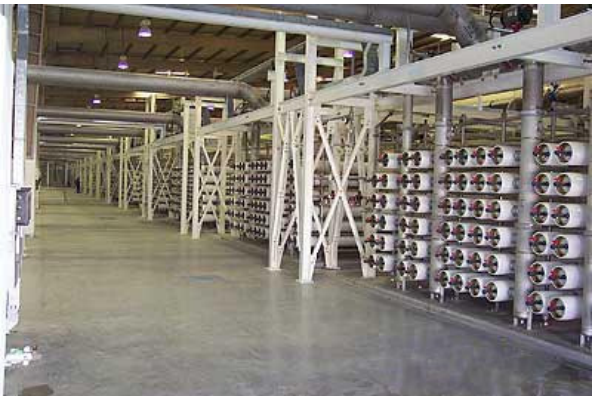
desalting of seawater plant using RO membrane in Kuwait desalination of seawater water purification technology
